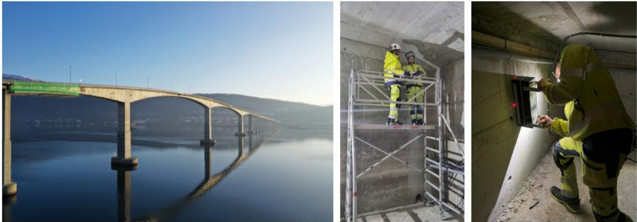
Figure 6 Practical challenges during NDT inspections of post-tensioned bridges, including access via scaffolding above water, confined interior spaces, and overhead scanning in constrained positions
