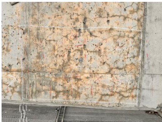
Figure 52 Surface cracking due to Alkali-Silica Reaction (ASR) observed on the Gisund Bridge
